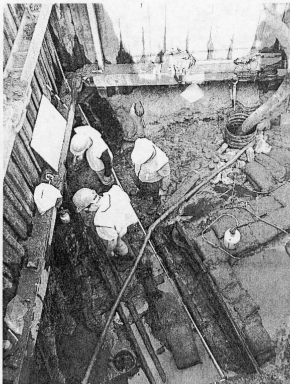
Deep in the caisson-protected hole, archaeologists used video cameras, sketches and measurements to record what will be completely lost after the road is completed. The watersoaked ground was the boat's salvation, the anaerobic environment preserving the wood.
